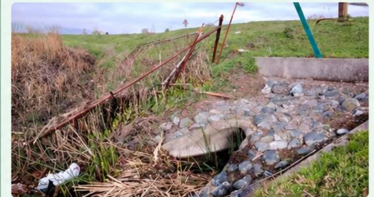
Outfall with vegetation overgrowth
