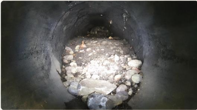
Clogged pipeline (Pole-camera inspection)
