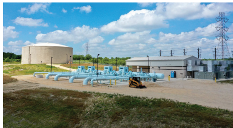
Vista Ridge Regional Supply Project infrastructure in Central Texas, supporting a new, drought-resistant water supply designed to serve the region reliably for decades.
