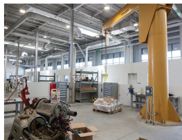
LEED-Gold Port of Long Beach Maintenance Facility
