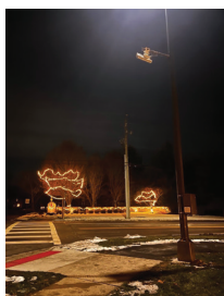
The SecurOS® Soffit provides dynamic LED illumination for pedestrians at the Brand Road crossing near Coventry Woods Drive in Dublin, Ohio.
