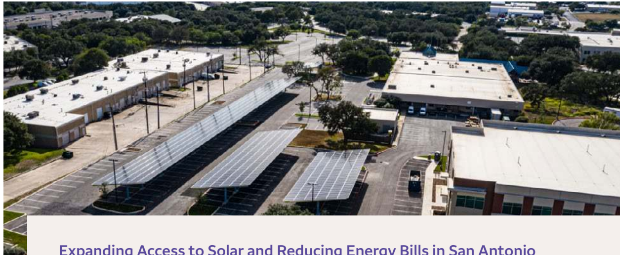
One of Big Sun Solar’s 12 canopy sites across San Antonio. Photo courtesy of Big Sun Solar.
