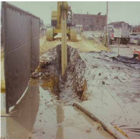
Construction of a slurry wall in progress on the Harbor Point site. (Photo courtesy of the City of Baltimore)
