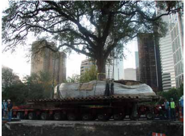
During excavation a number of live oaks were carefully relocated to another section of the park site.
