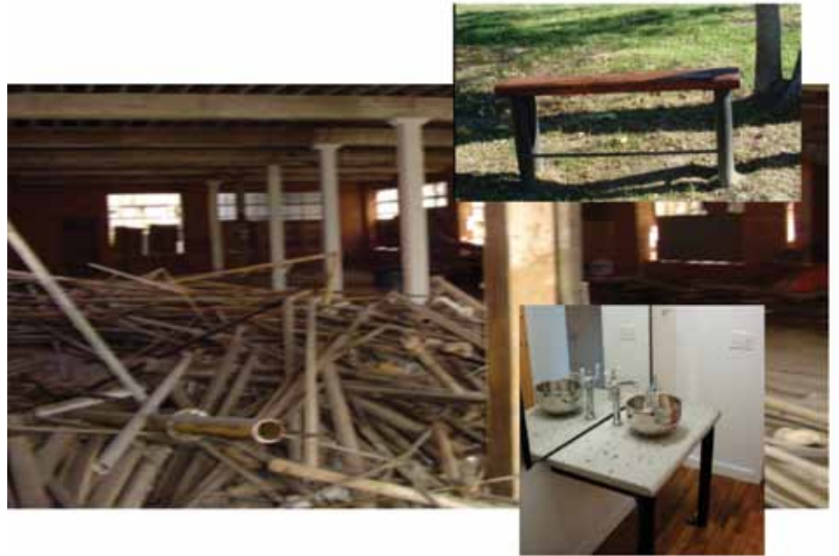
Old sprinkler pipes have been recycled into custom vanities, bars, guardrails, and outdoor benches. (Photos courtesy of Mica Village Partners, LLC)
