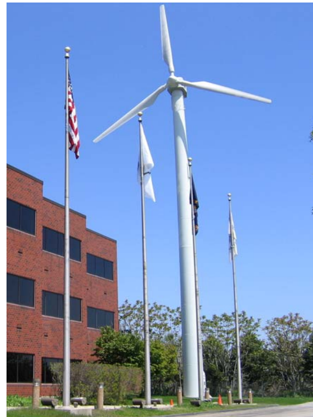
IBEW Local 103 100 kW Turbine
