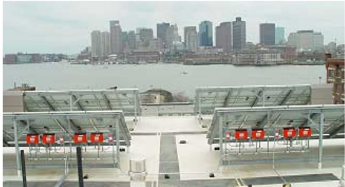
Maverick Gardens Affordable Housing Photo Voltaic System
