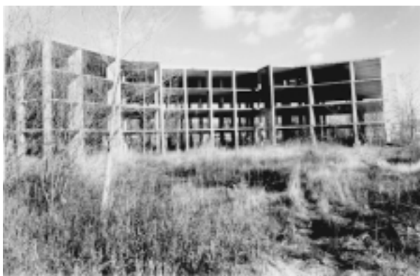
CAPTAIN'S COVE ABANDONED STRUCTURES: These buildings have been demolished and the site is being cleaned up. A hotel conference center with associated retail will be built here soon. (Photo courtesy Jambhekar Strauss Architects PC)
